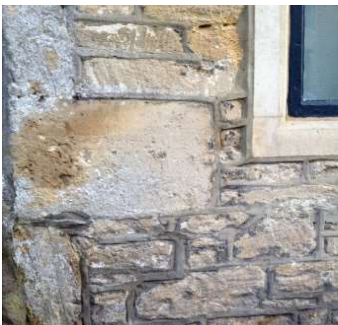
Cement rich ribbon pointing in Pickwick Street
